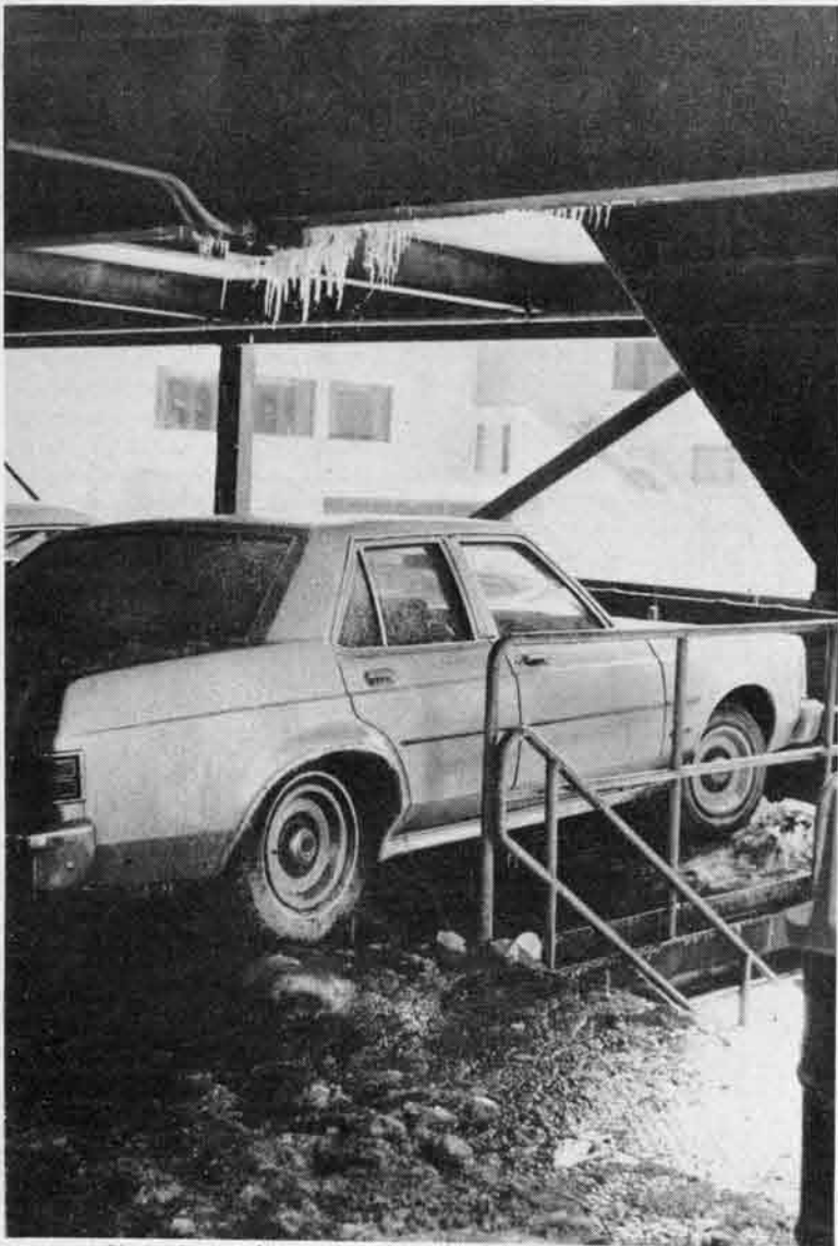
POOR FOOTING: Dripping water from the ceilings of the parking garages have created hazardous ice conditions [photo by Dale Nelson].
